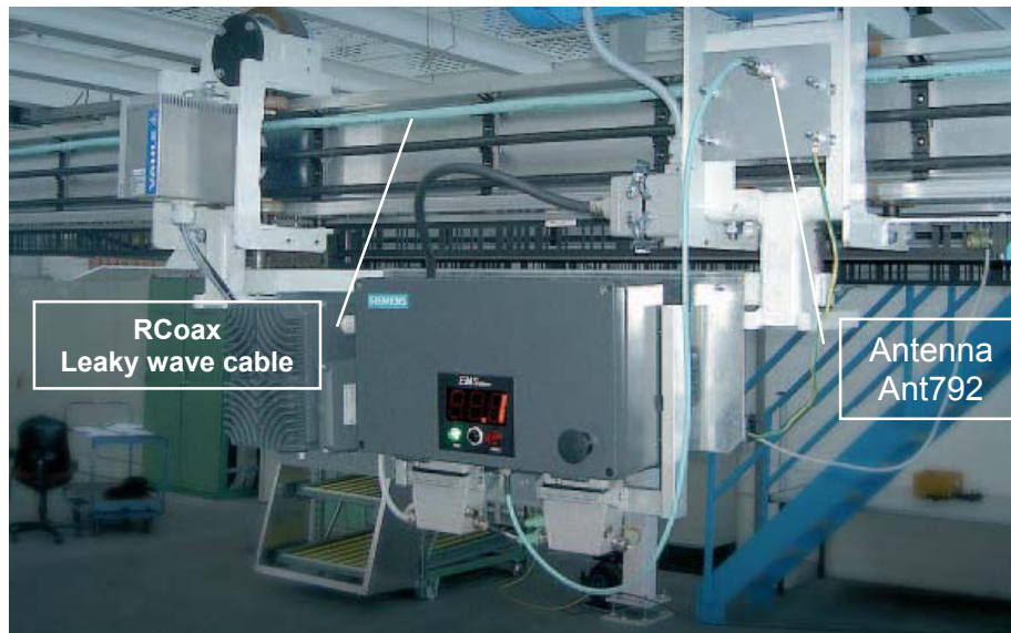
Monorail conveyor as an example for the IWLAN/RCOAX application
